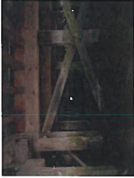
Photo 2.9 – Downtown Riverview Pier - Typical Pier Substructure The pier structure was observed from the deck level on foot and from below by kayak.
