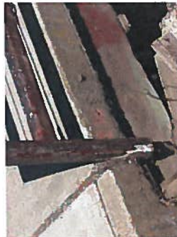
Photo 3.39 - Downtown Fishing Pier - Pier Access Handrail
