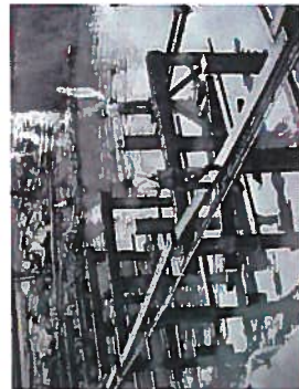
Photo 2.5 – Downtown Riverview Pier - Pier Pile Bent Construction (Date Unknown but assumed 1947 or earlier)
