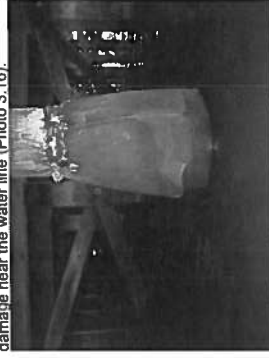
Photo 3.15 – Downtown Riverview Pier - Pier Pile with Wrap
