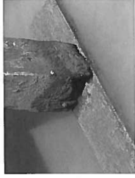
Photo 3.16 – Downtown Riverview Pier – Pier Pile Damage
