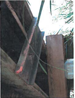
Photo 3.10 - Marina Fishing Pier - Light Pole Base Connection
