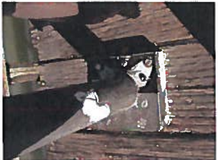
Photo 3.9 - Marina Fishing Pier - Damaged Light Pole Cover
