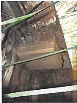
Photo 3.12 - Marina Fishing Pier - Electrical Conduit
