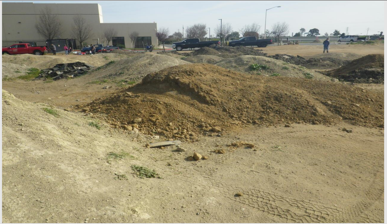
Photograph 34 – View of Soil Piles on Northern Portion of Parcel 56, 3215 E. 18 th Street
