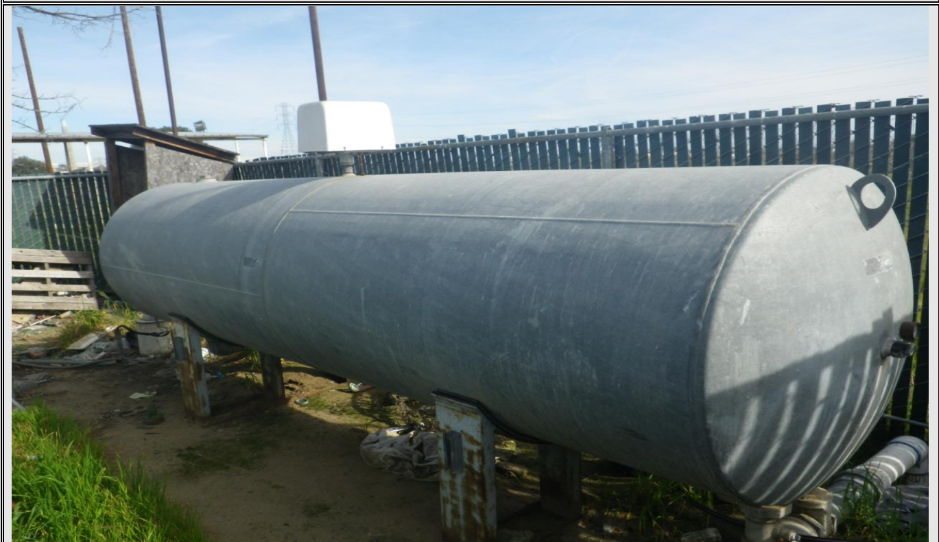
Photograph 32 – View of Water Tank, 2901 E. 18 th Street, Parcel 86
