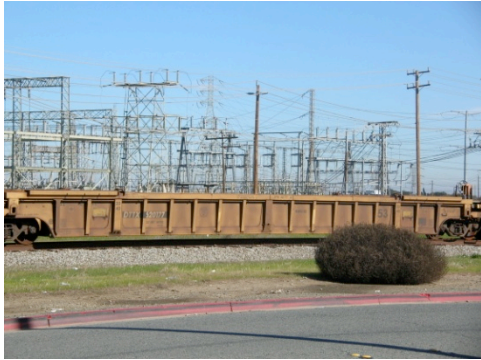
Hillcrest Avenue Substation and rail line
